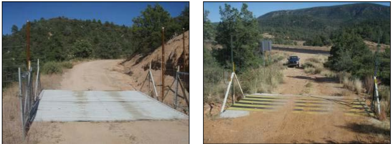
Figure 4.3. Dual cattle guard (left) and ElectroBraid™ ElectroMat (right) designed to allow lateral road access for vehicles while preventing wildlife from entering the fenced SR 260 ROW.
